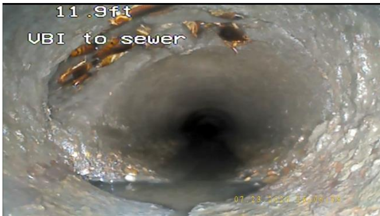
Section of damage or pipe offset, crack at base, approx. 8' from E. Yard cleanout
