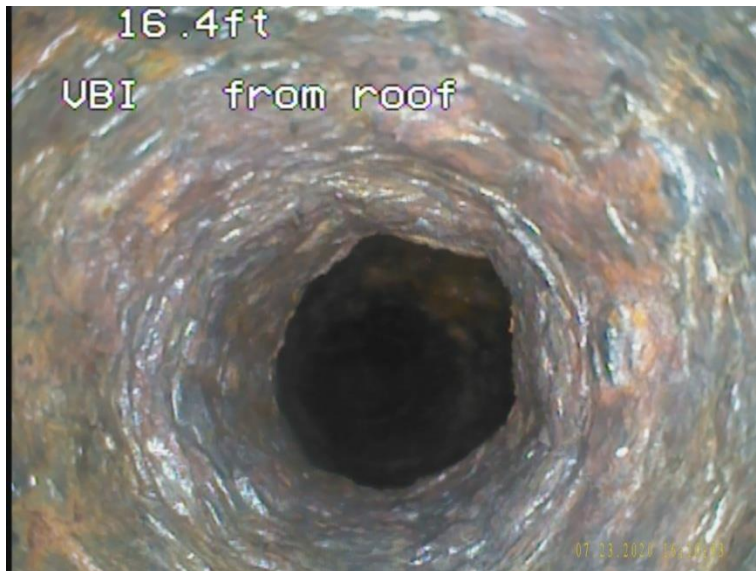
General view of rusting at cast iron piping
