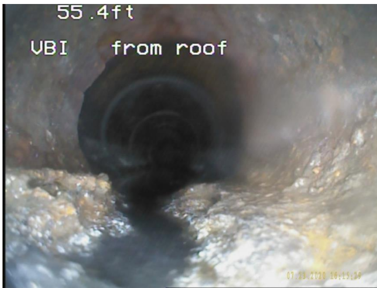
Debris at cast iron piping
